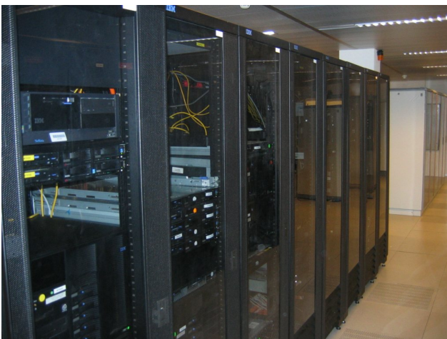
Data centre: AI's "immaterial" world remains an infrastructure of metal, cables, electricity, water and territory. Photo: Wil Weterings, public domain, Wikimedia Commons.
