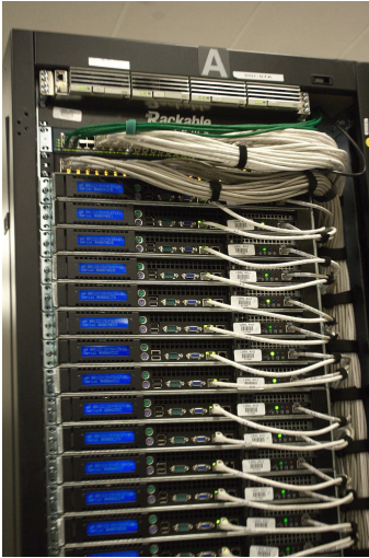
The rear of a server rack at the NERSC computing centre: the material reality of digital infrastructure. Wikimedia Commons, CC0.
